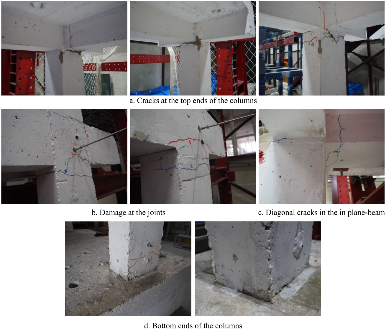
Figure 7. The damage distribution observed in the scenario without pounding effects
