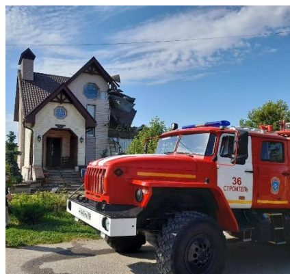
Figure 16. Example of the effects caused by attack elements neutralized by the air defense system (Governor of Belgorod, 2024).
