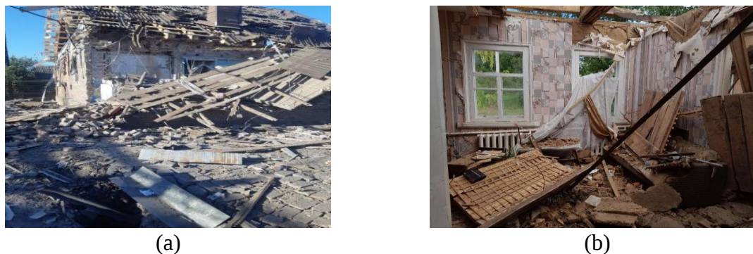
Figure 12. Examples of Severe Damage are a) Severe exterior damage to the structure and b) Severe interior damage to the structure (Governor of Belgorod, 2024).
