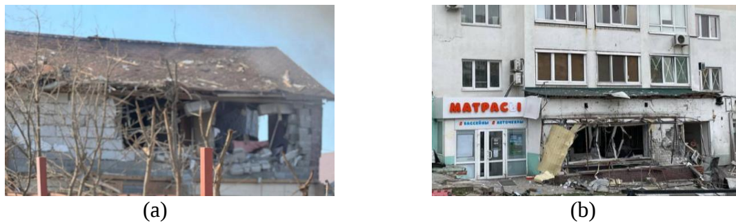
Figure 11. Examples of Moderate Damage are a) Collapse of non-load-bearing wall and roof damage and b) Damage to facade, windows, and doors along with porch and mechanical systems damage (Governor of Belgorod, 2024).
