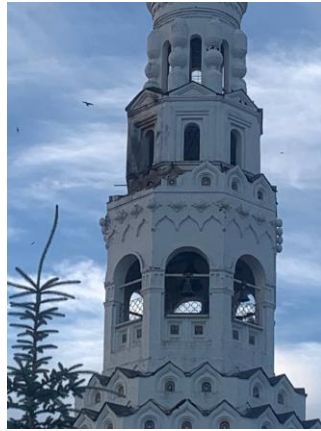
Figure 15. Example of damage caused by UAV to structures (Governor of Belgorod, 2024).
