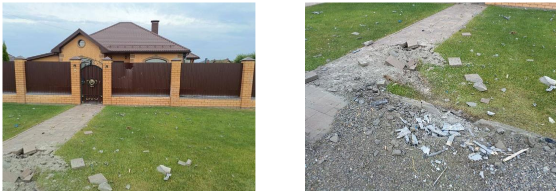
Figure 9. An example of attacks that did not cause structural damage (Governor of Belgorod, 2024).
